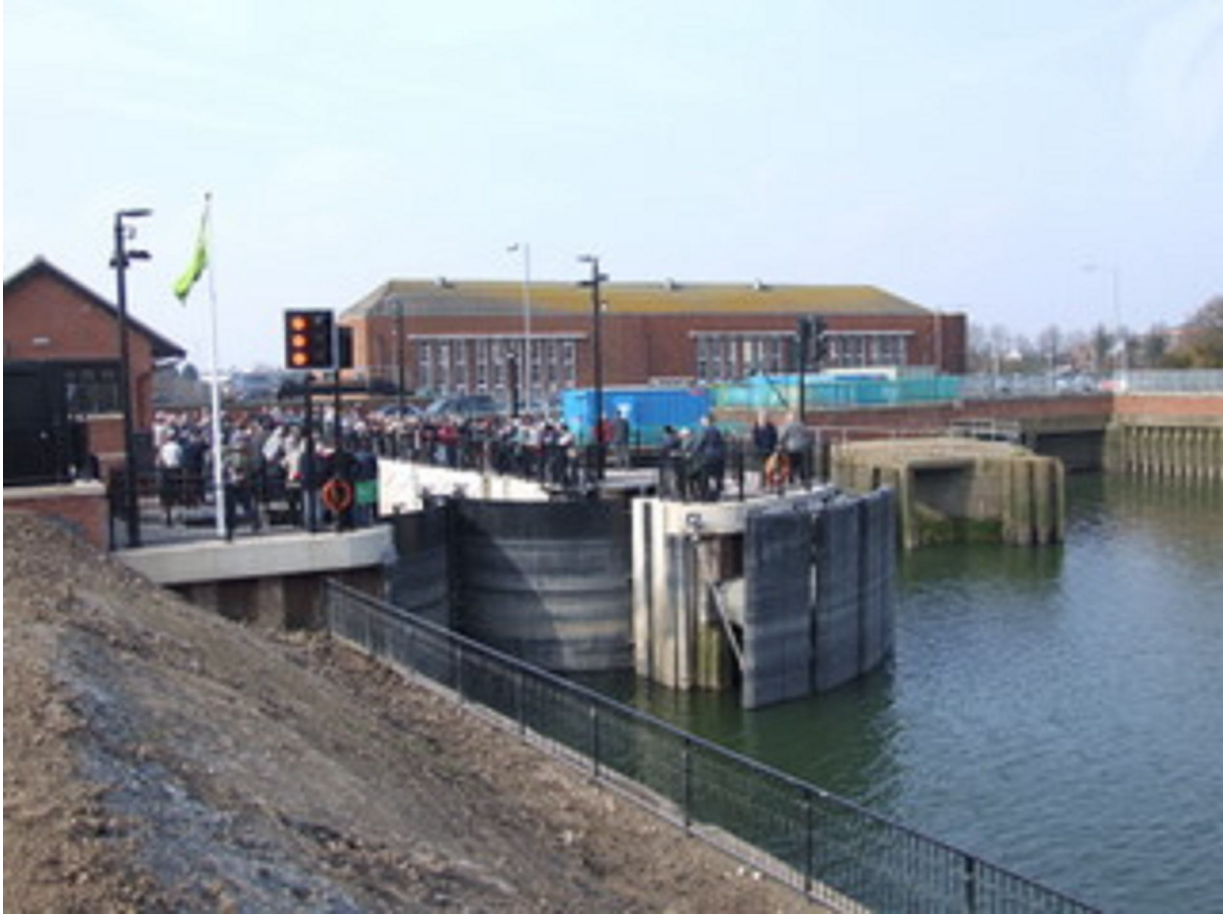
The new lock from the seaward side. In the background (right) is the Black sluice Pumping Station, first built in 1946 but extended in the 1960s.
