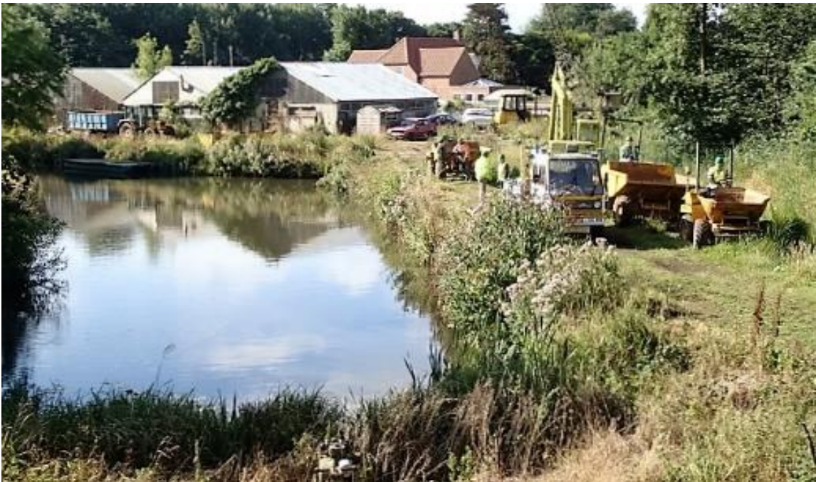
A line up of plant for the day at Bacton Wood – three dumpers, one digger and one lorry. The plant was for use on the North Walsham bank opposite Pigneys Wood where the lorry was parked by the new sluice with the tools and grass seed for completion of the seeding on the north west bank.
