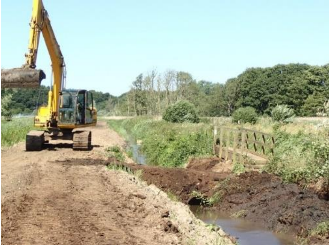
The work of the Old Canal Company and the volunteer workers carries on. This picture was taken on 14 August at Pigneys Wood and shows the digger which has just installed a large pipe on the back soke on the right as a prelude to establishing a pedestrian crossing.
